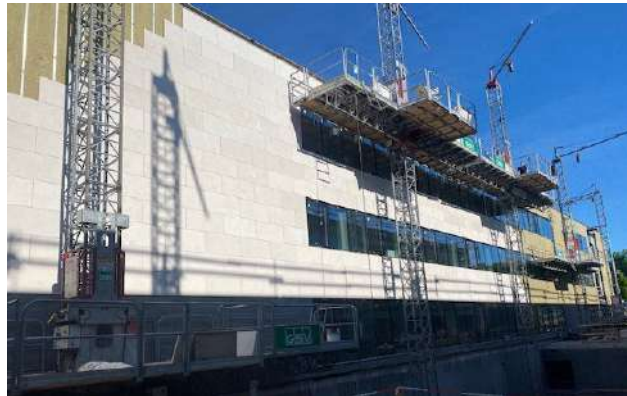
Project: JYSK HEADQUARTERS Location: Brabrand, Denmark Architect: ARKITEMA ARCHITECTS Contractor: Dybdal Contracting Year: 2021
